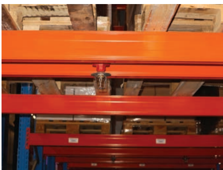
In Rack sprinklers
