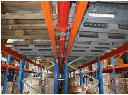
In Rack sprinklers
