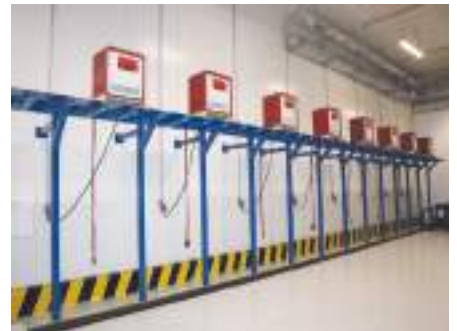
Battery charging room
